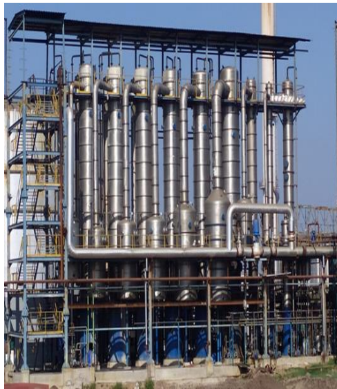
I st Stage Evaporation (Falling Film)
