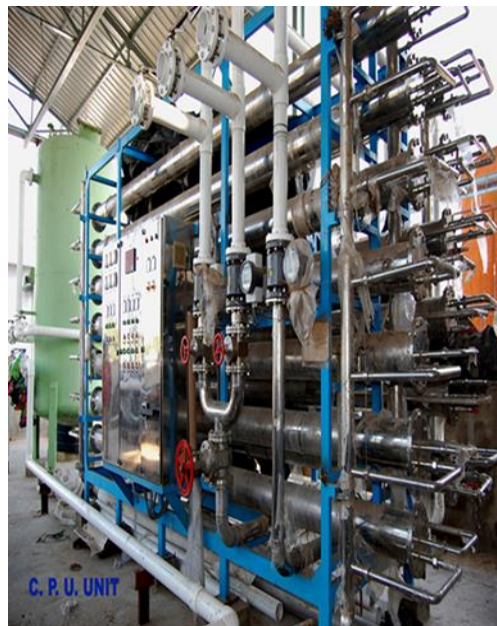
Condensate Polishing Unit (RO System)
